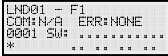
Figure 37: Hall Lantern Status
