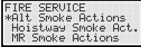
Figure 257: FIRE SERVICE Menu – Alt Smoke Actions, Hoistway Smoke Actions, MR Smoke Actions
